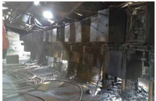
Medium voltage switchgear destroyed by arcing fault prior to installing Arcteq IEDs and arc protection systems.
